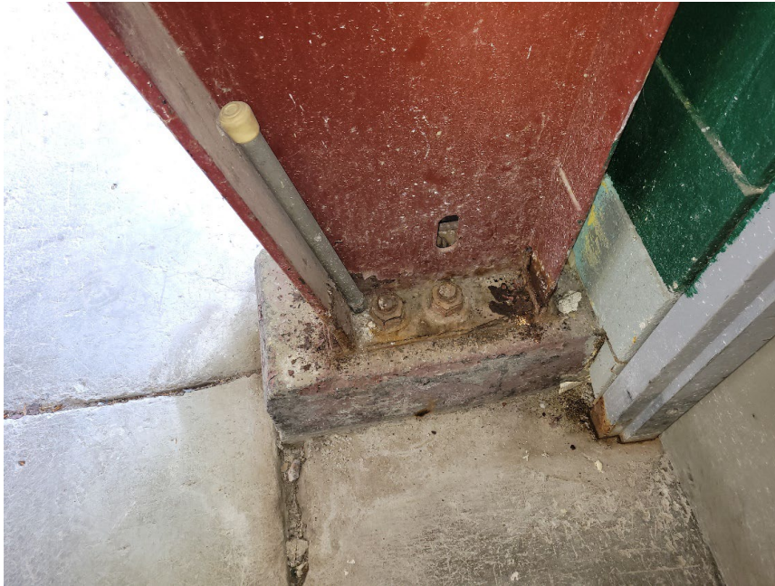
Figure 1 - Corrosion at Base Plate of Column by Overhead Door
