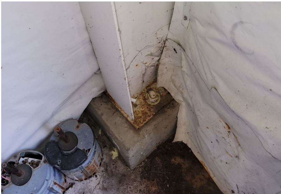
Figure 2 - Corrosion at Base of Gable Column by Overhead Door
