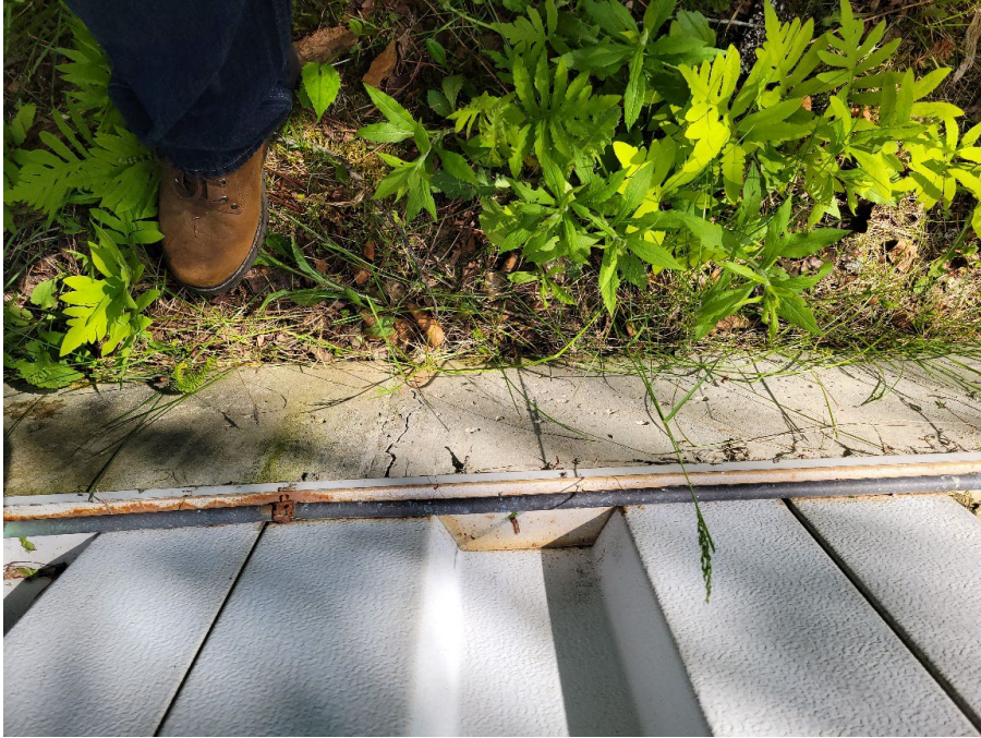
Figure 6 - Cracks in foundation at exterior
