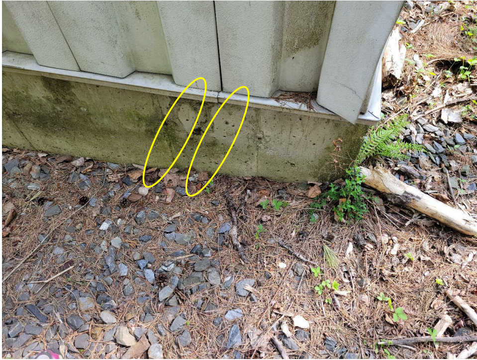
Figure 5 - Cracks in foundation at exterior
