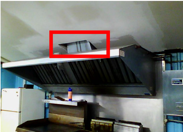
Air leakage was observed around this duct penetration for the kitchen exhaust.
