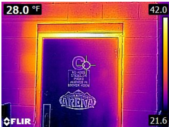
Warm air is visible around the perimeter of the door.
