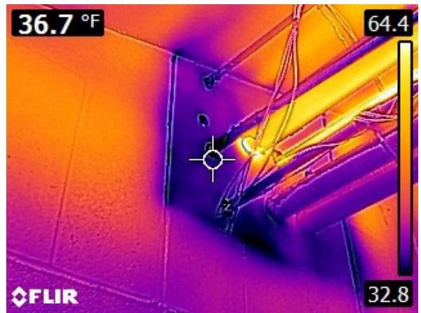
Penetration in conditioned space "E", these penetration lead to the unconditioned vestibule.
