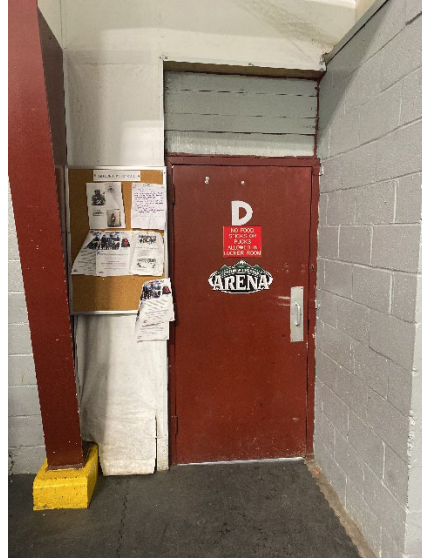
Looking at a typical door separating the conditioned spaces such as the locker rooms and bathrooms from the arena. No door bottom is present, a gap is visible at the base of the door.
