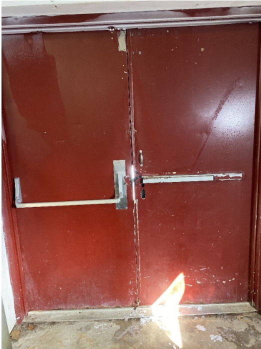
Daylight is visible at the latch connection of these door doors.
