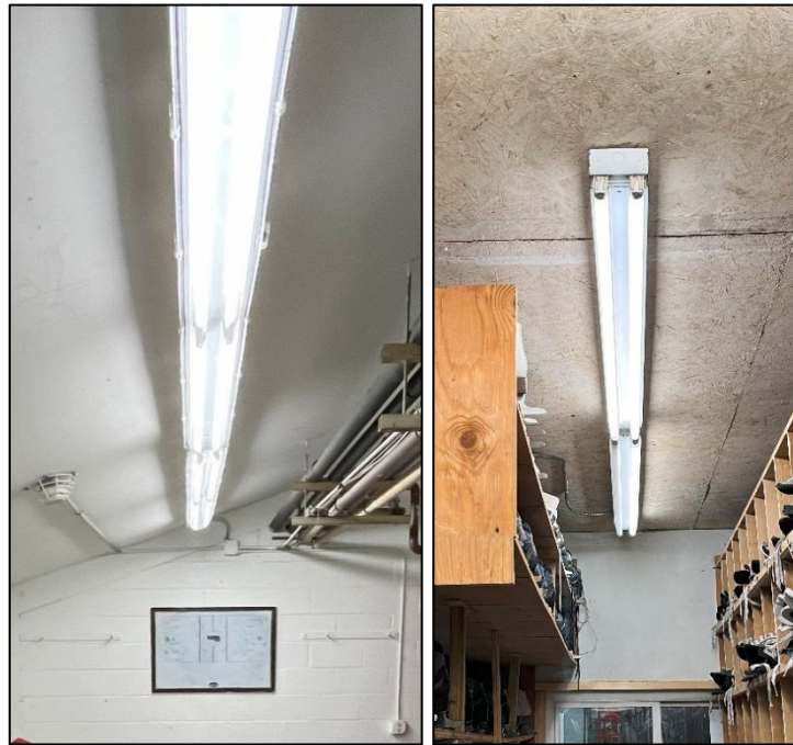
Figure 2: Example lighting, a new LED fixture with cover (left), and an older T8 fixture (right)
