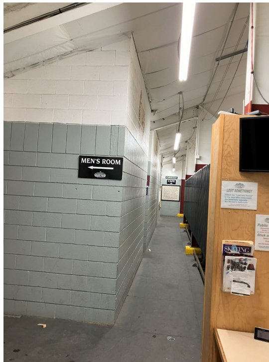
Looking down a section of CMU wall that separates the bathrooms and locker rooms from the unconditioned arena space.
