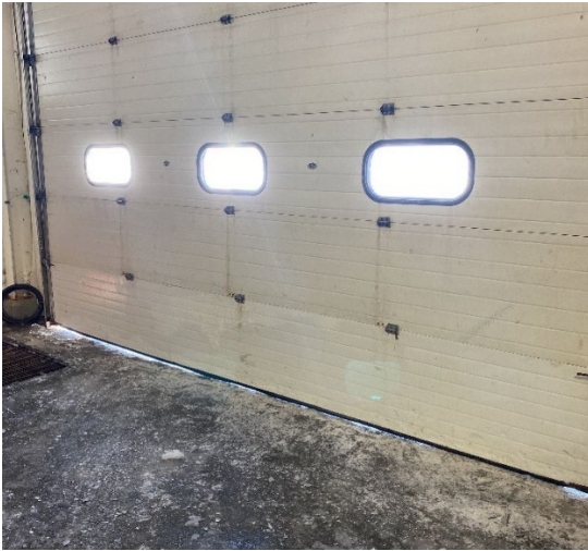
This overhead door does not seal well at the bottom, this is partially due to ice build-up.
